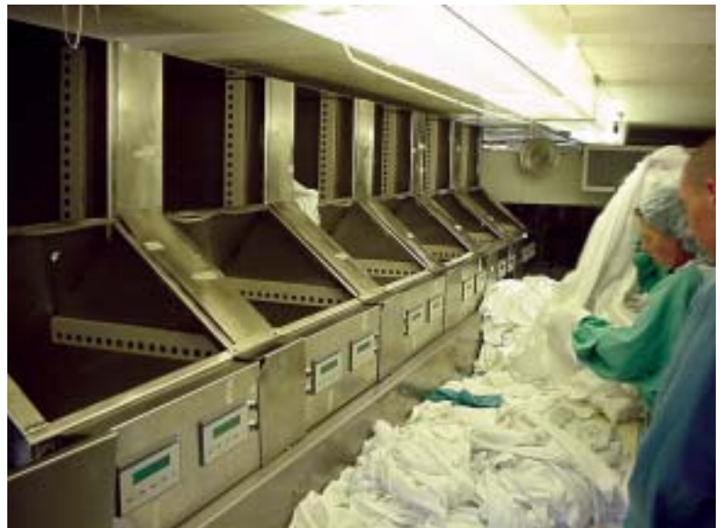
The soil room is the entrance goods follow into the plant.
